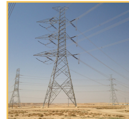
GS - IRRQAA BSP Arabia 380kV Line 180km hardware & fittings and damping system.
