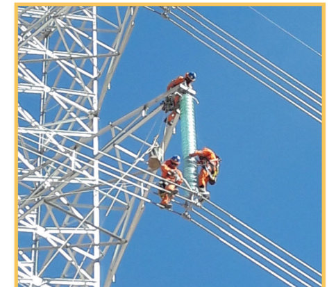
Bangladesh - Patuakhali - Gopalganj Transmission line 400kV four-bundle TL HTLS ACCC conductor.
